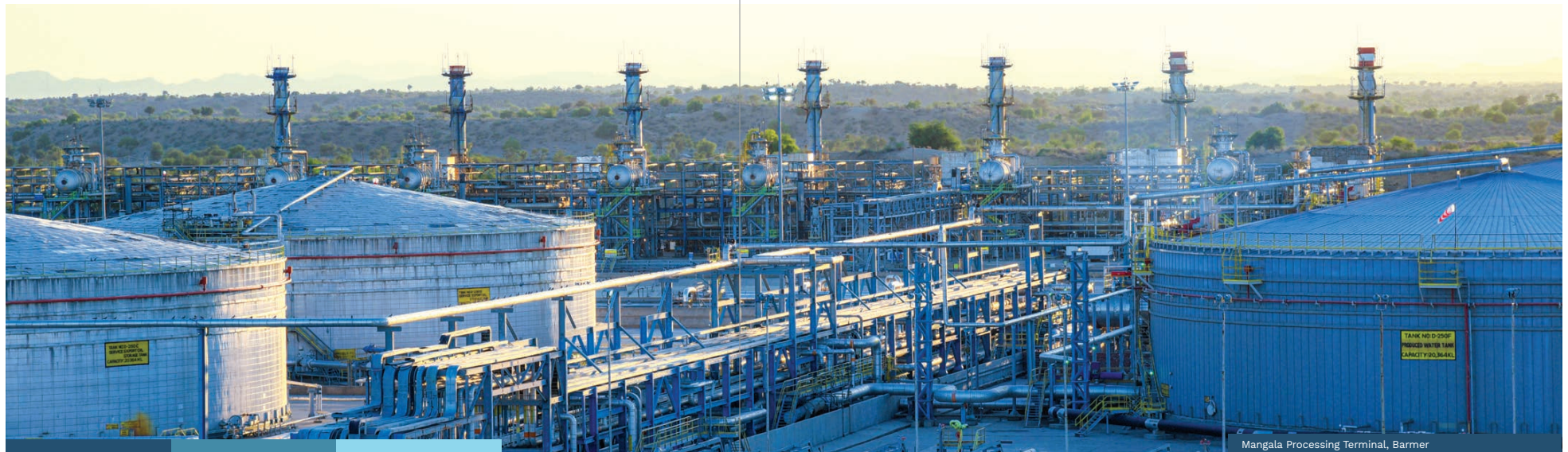
Mangala Processing Terminal, Barmer
