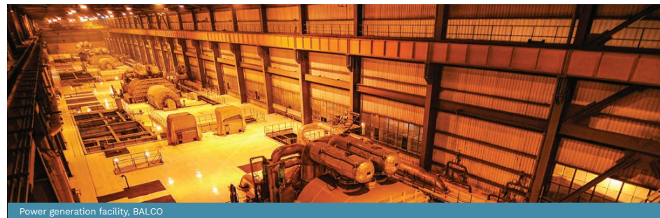
Power generation facility, BALCO
