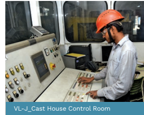
VL-J_Cast House Control Room
