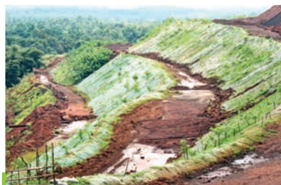
Below: Geotextile laid on dump slopes for dump stabilisation at Codli mine
