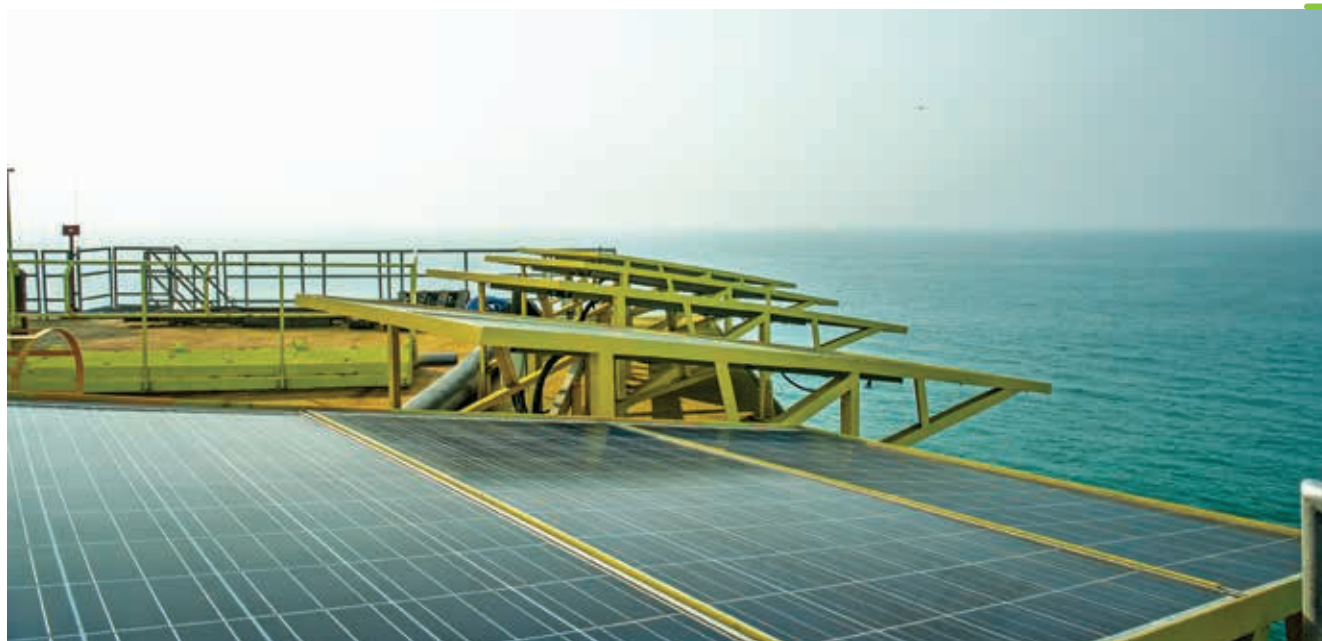
Top: Our offshore well-pads are powered by renewable energy.
