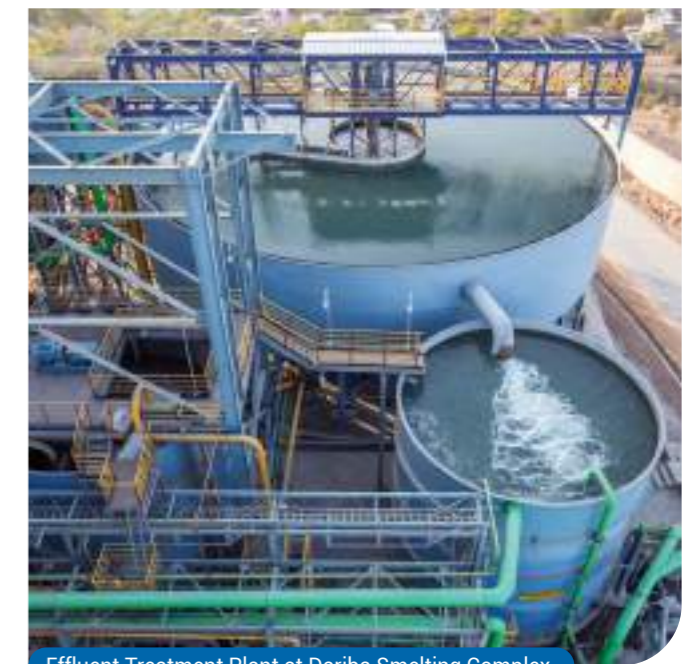
Effluent Treatment Plant at Dariba Smelting Complex
