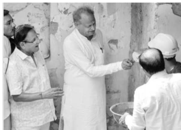
Rajasthan CM Ashok Gehlot launches renovation works at a stepwell under Indira Gandhi Shehri Rozgar Guarantee Yojana, in Jaipur on Friday. PHOTO: PTI
