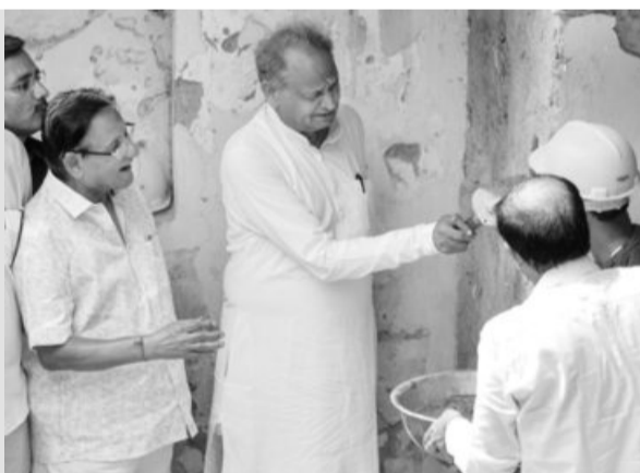
Rajasthan CM Ashok Gehlot launches renovation works at a stepwell under Indira Gandhi Shehri Rozgar Guarantee Yojana, in Jaipur on Friday. PHOTO: PTI
