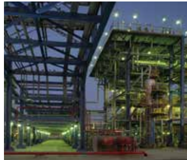
Left: Rajasthan: Raageshwari Gas Terminal
