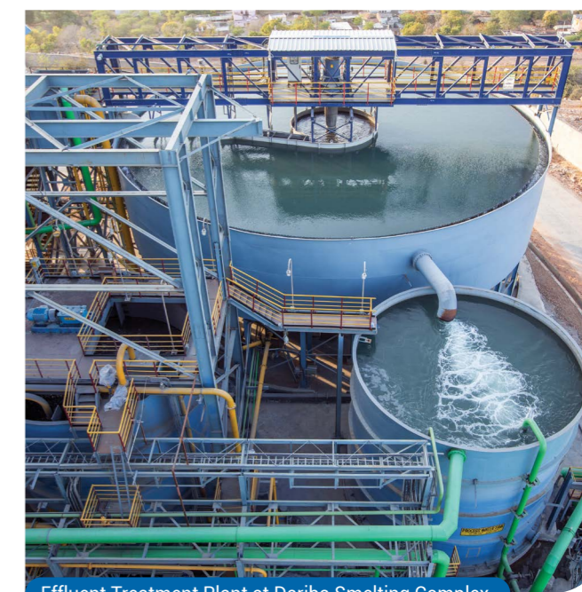
Effluent Treatment Plant at Dariba Smelting Complex
